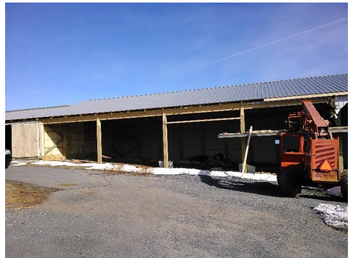
One of the new sheds that has been built during the winter.
