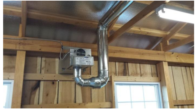
Ventilation system in Blacksmith Shop
